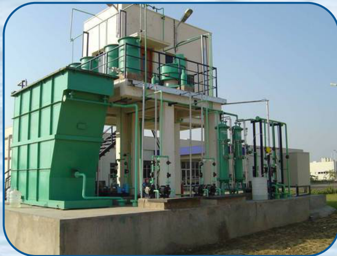
EFFLUENT TREATMENT PLANT
